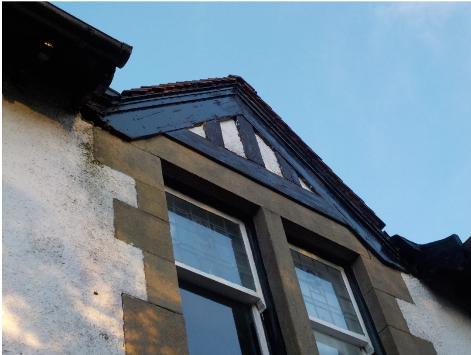
Photograph No.6 – Decaying decorative timber above window
