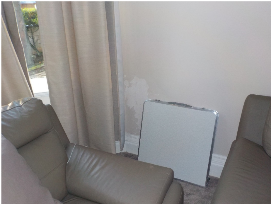
Photograph No.16 – Front left-hand ground floor living room – flaking of paintwork
