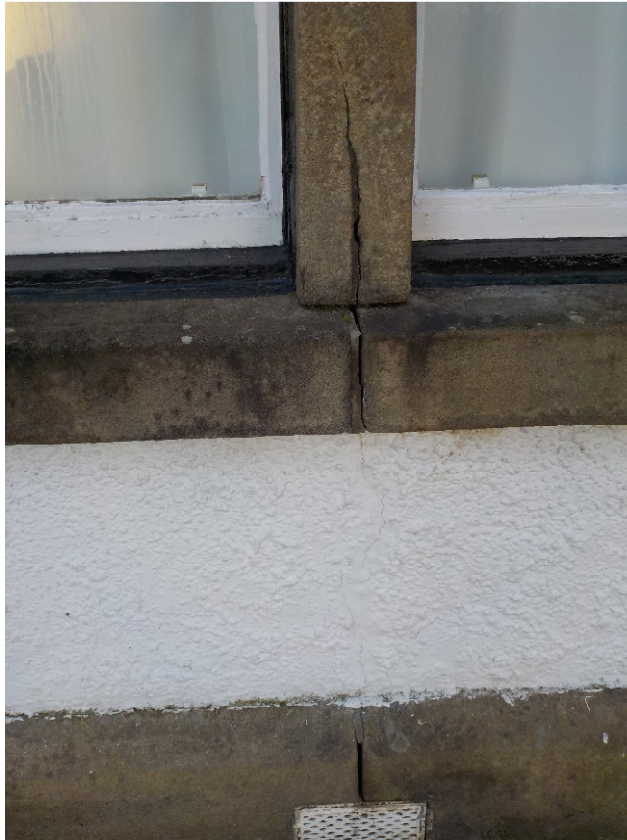
Photograph No.2 – Splitting in stone mullion
