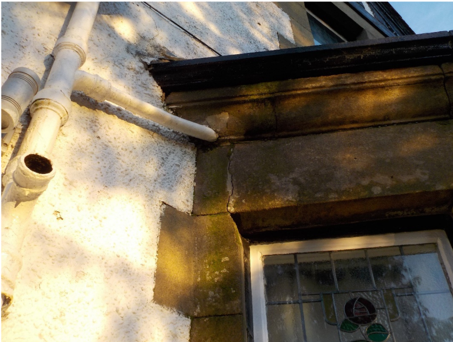
Photograph No.4 – Cracked stone lintel
