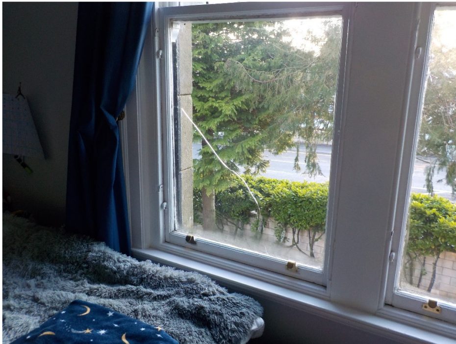
Photograph No.17 – Front, first floor right-hand window – cracked glass
