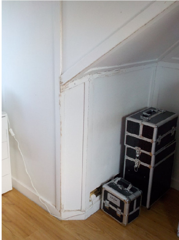
Photograph No.19 – Attic area – damp staining on finishes
