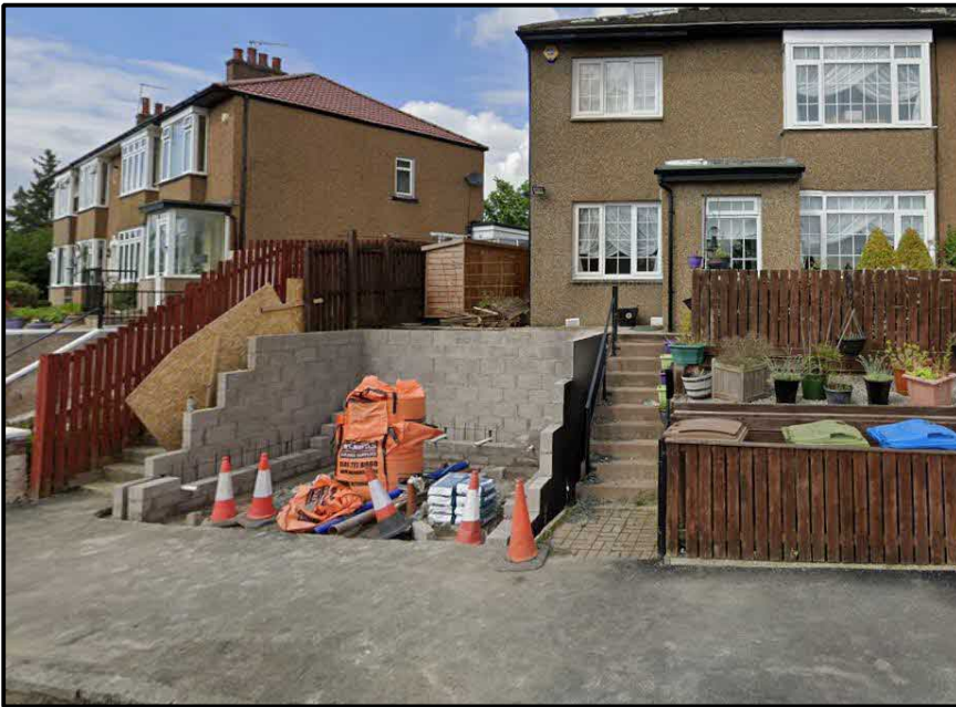
Under construction front driveway with retaining wall and steps to front of house door.
