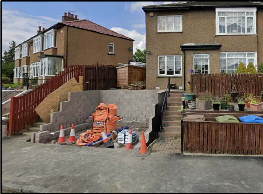
Under construction front driveway with retaining wall and steps to front of house door. Elevated to similar level as proposal
