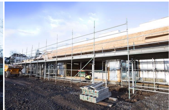
• Overlee Nursery, Clarkston
