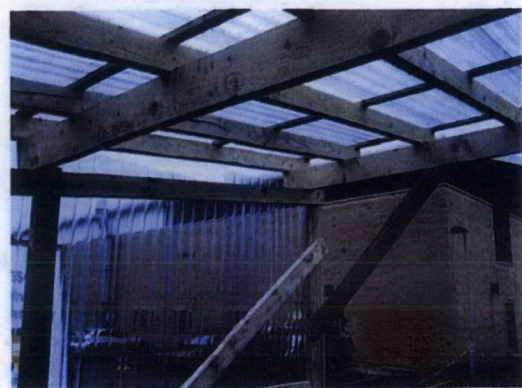
Corner Detail of Valeting Shelter showing cross bracing and diagonal supports to main frame.
